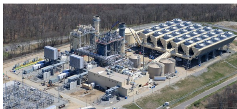
CPV Towantic Energy Center | CPV
